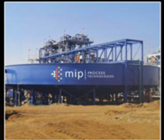
26m \phi Thickener in operation
