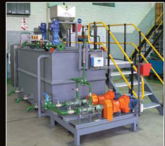
MIP-200 Flocculant Plant
