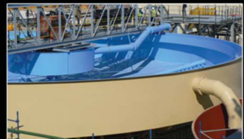
26m \phi Thickener installation
